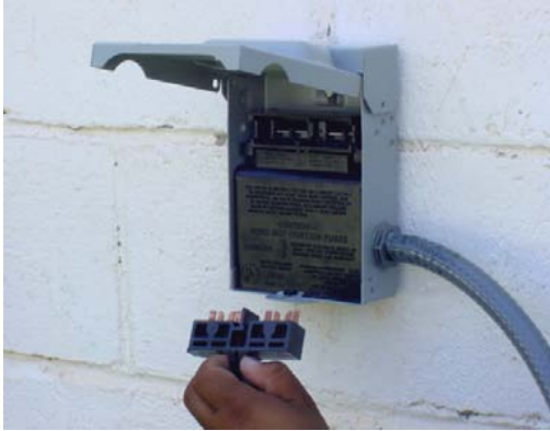
Disconnect All Electricity Before Servicing To avoid Electricity DANGER Of Serious Injury or Death
