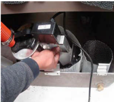
Remove pump & clean screen.
